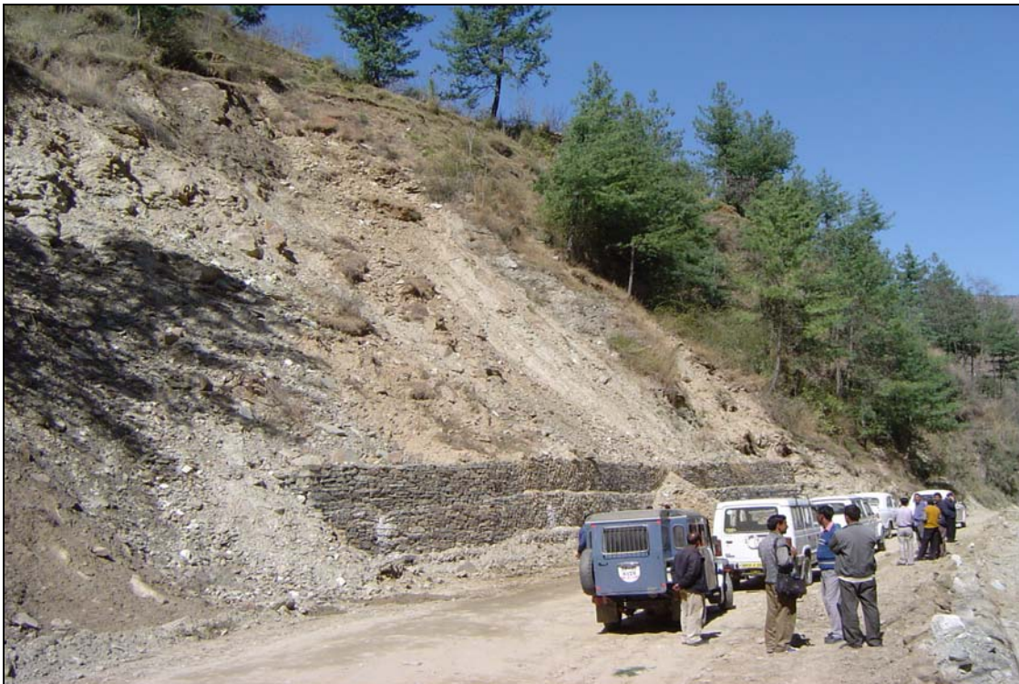
Plate 3. An Example of a Gabion (wire crate) Wall - Failure such as this need Additional Treatment.
