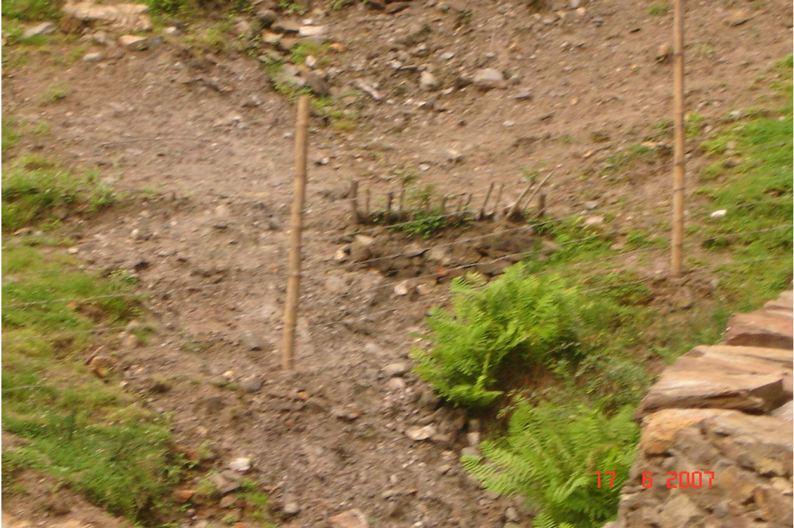
Plate No. 5: Vegetated palisade construction in the Sundali nala and performance of the growth after 6 months.
