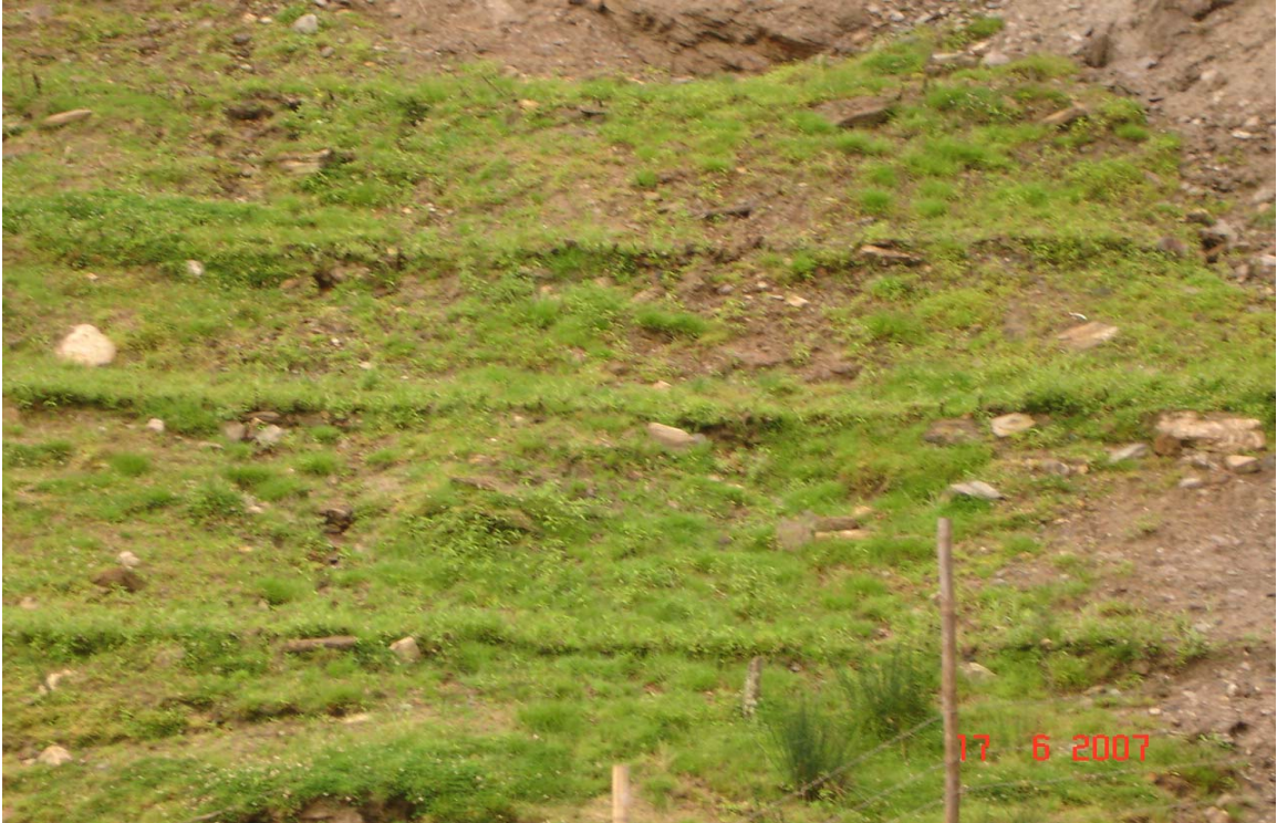
Plate No. 3: Several rows of brushlayering works in Sundali nala gully and performance of the growth after 6 months of construction.
