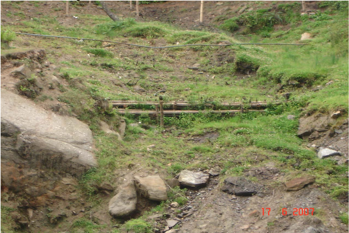
Plate No. 4: View of the upper part of Sundali nala gully showing bamboo cribwall construction after 6 months of construction.
